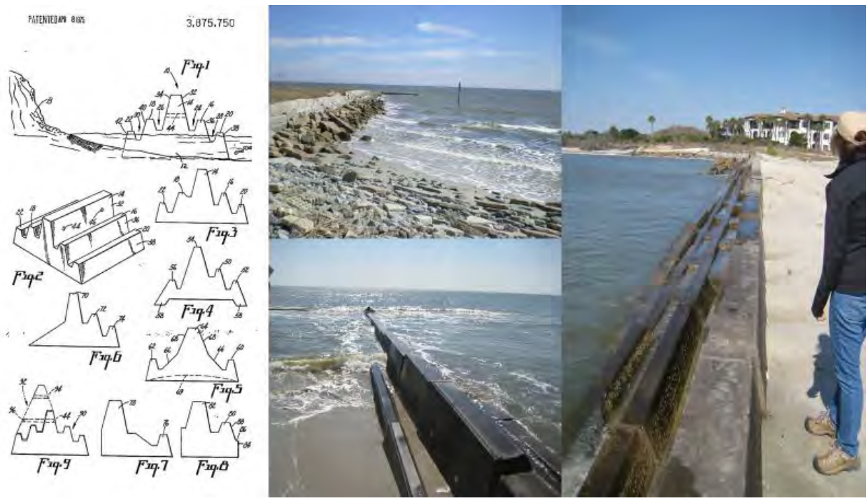
Figure 6 Original sketches of Campbell modules (left) from the patent and photos of the South-end groin (March 2014)
