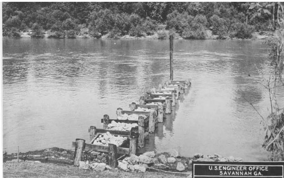
A completed pile dike used for channel contraction Augusta. Note the inner core of brush fascines topped by a layer of rip rap stone, 21 September 1935. (Savannah District, Corps of Engineers)
